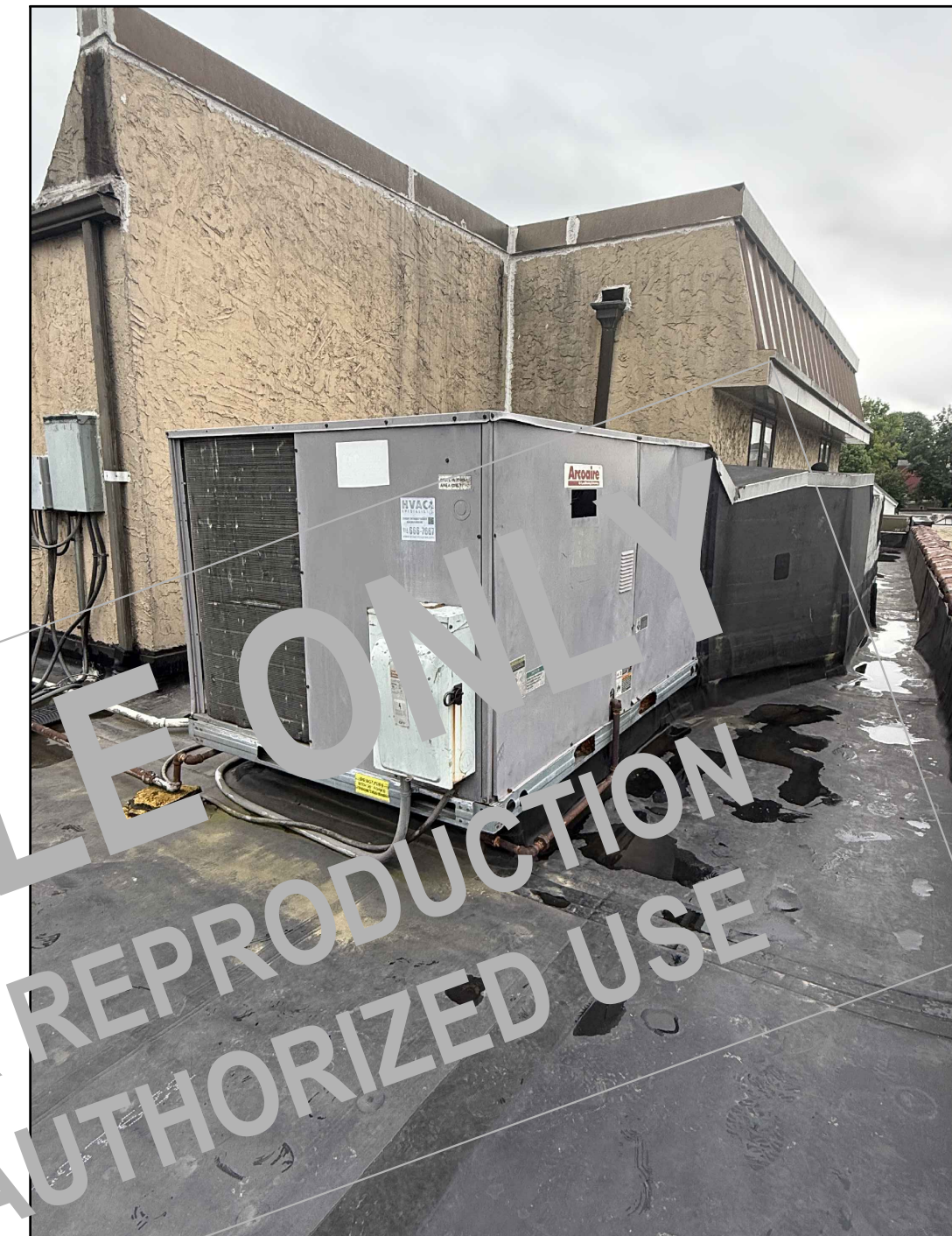
EXISTING ROOFTOP UNIT
